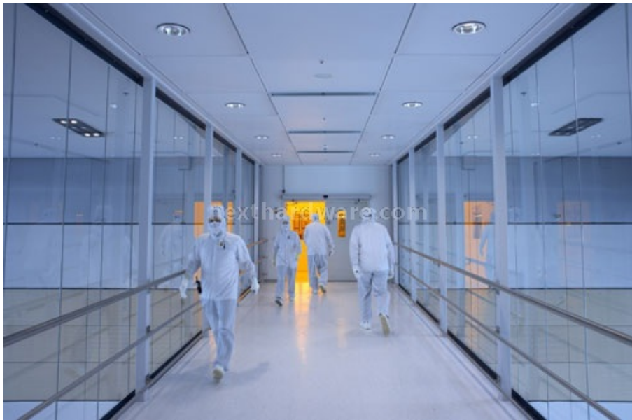
The Foundry Company will proceed with an upgrade of the first AMD Dresden fab, connected by a walkway to the second fab.
